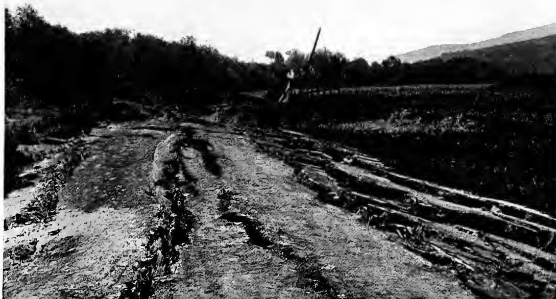
A. Lurching of ground toward Salinas River and consequent collapse. Near Spreckels. A. C. L.
